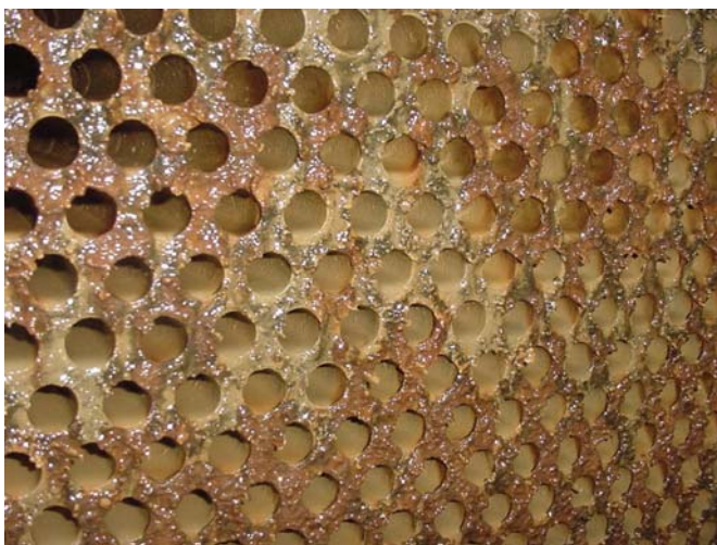
Condenser tubes – tube sheet after one (1) year of NCD treatment
