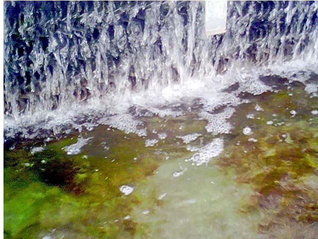
Cooling tower basin – algae and deposits
