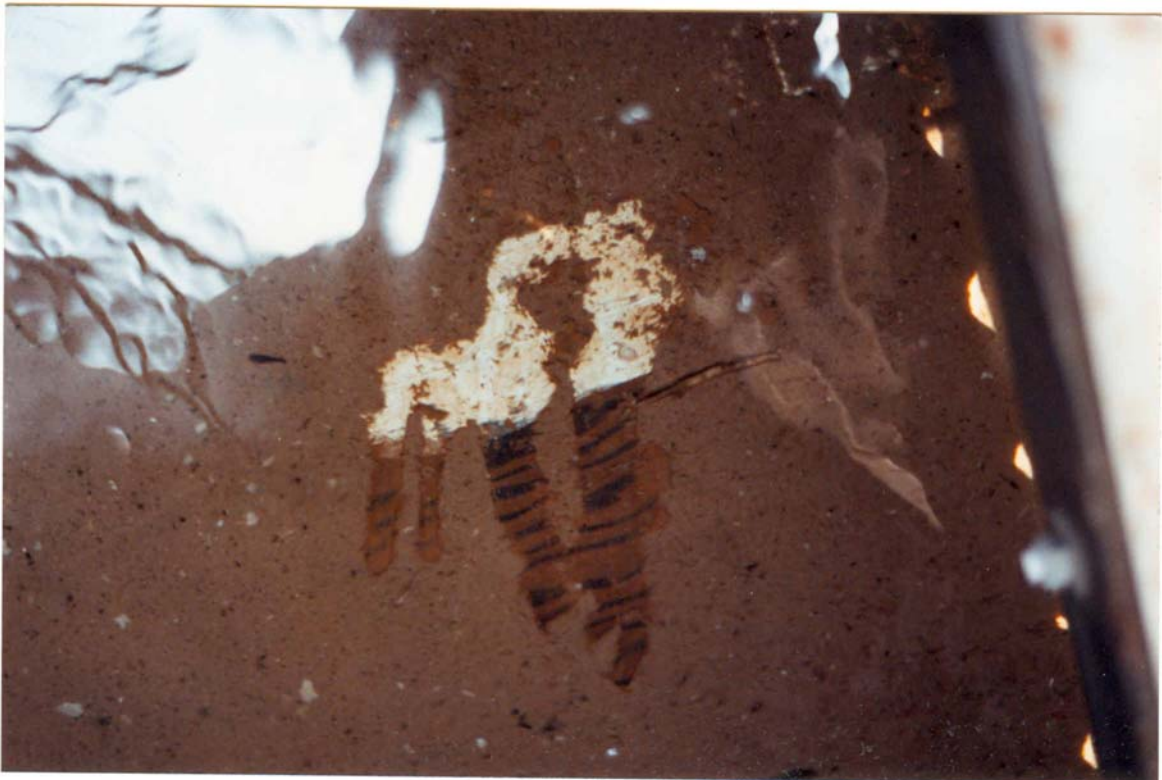
COOLING TOWER BASIN
