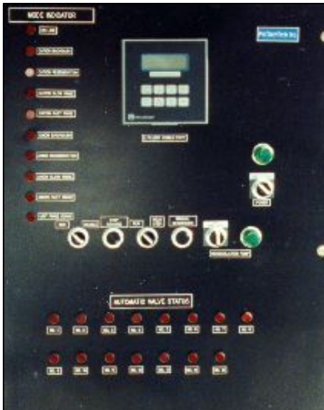
PCT manufactured ion exchange unit control panel.
