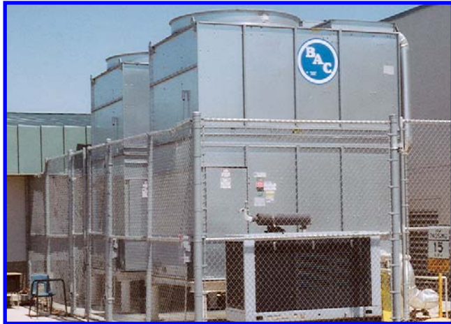
Typical HVAC Cooling Tower Installation
