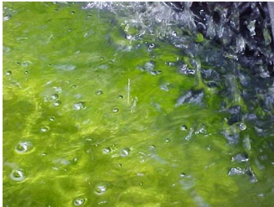
Algae Growing in Cooling Tower Basin
