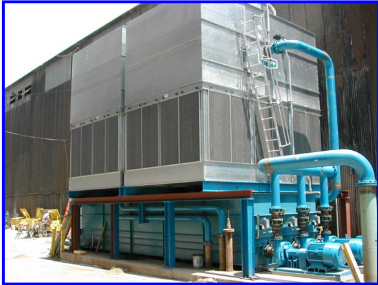
PCT Supplied Cooling Tower System – Steel Mill
