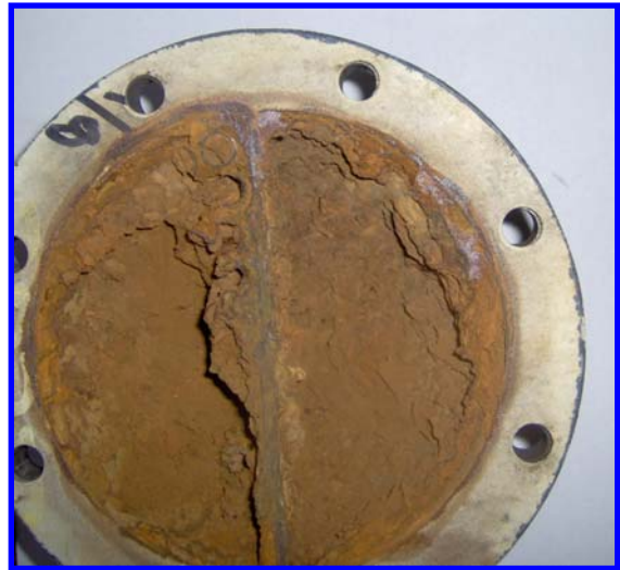
Corroded Steel Condenser End Bell
