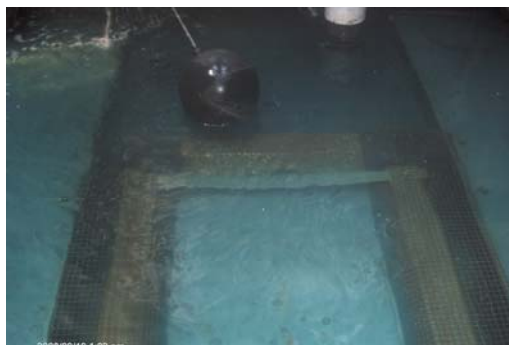
Scale Free Cooling Tower Basin
