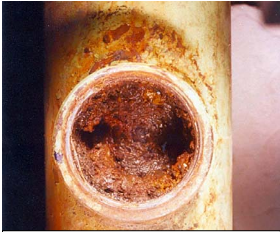
Outlet of Electrostatic Device Corrosion Products Deposit (Rust)
